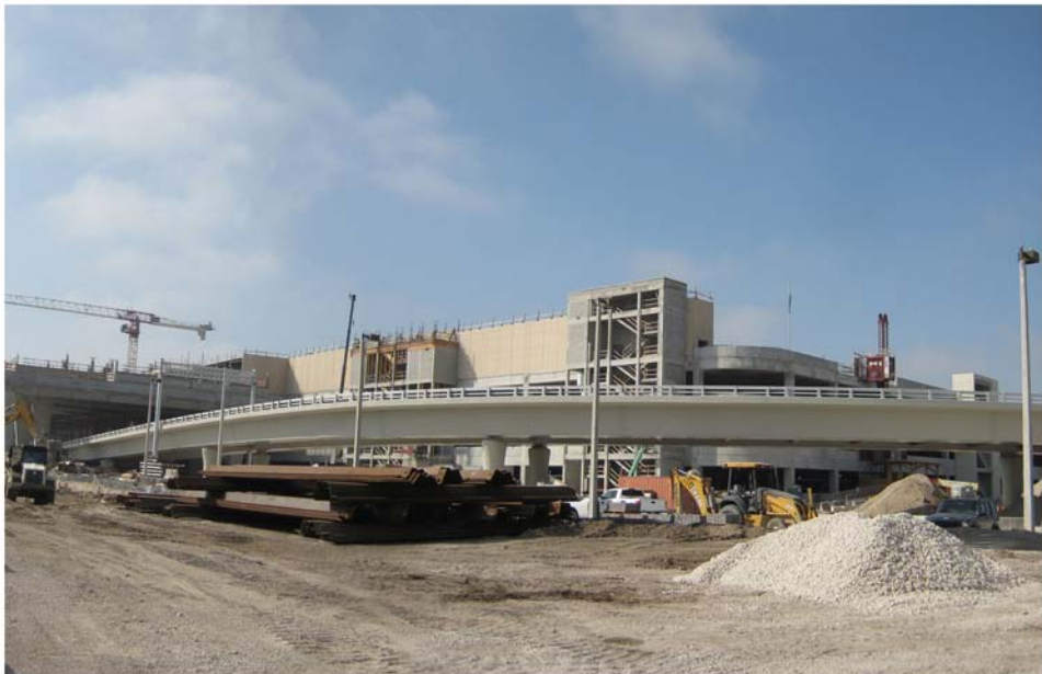
Miami Intermodal Center Construction: Progress Photo February 13, 2009 Rental Car Center (RCC): FM # 249937-5 / MTAR FM: # 249937-4 View of MIC Terminal Access Road Bridge 10-A and RCC beyond
