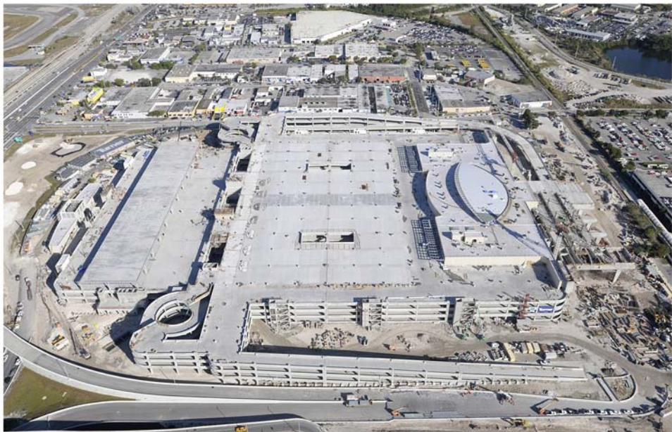
Miami Intermodal Center Construction: Progress Photo January 27, 2009 Rental Car Center (RCC): FM # 249937-5 Northwest View of RCC Construction Site
