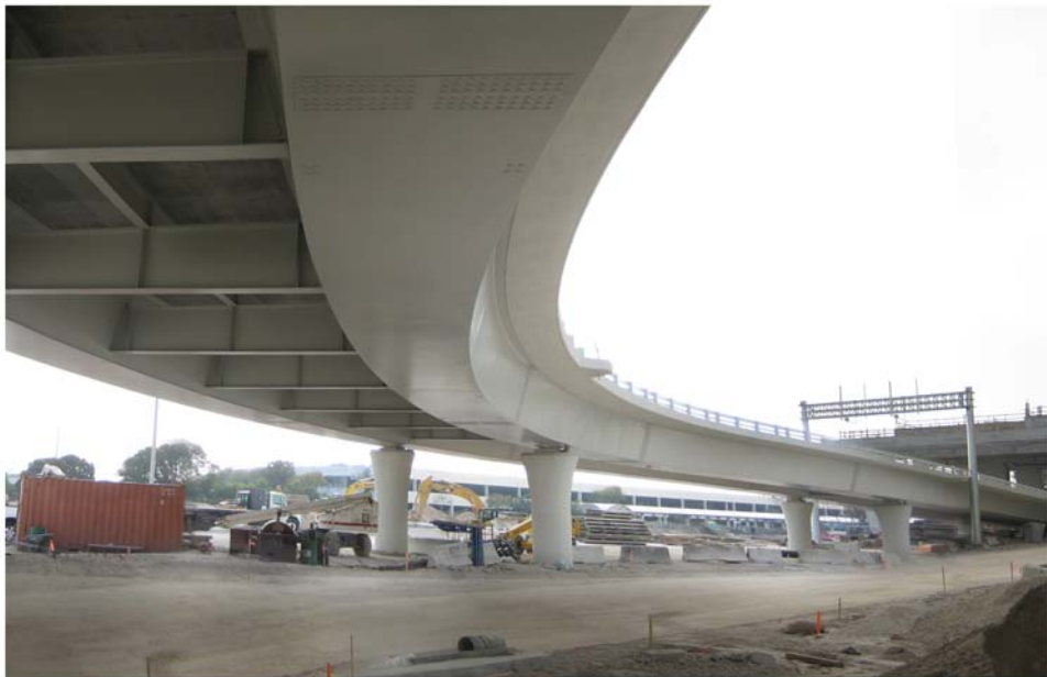
Miami Intermodal Center Construction: Progress Photo February 13, 2009 Rental Car Center (RCC): FM # 249937-5 / MTAR FM: # 249937-4 View of MIC Terminal Access Road Bridge 10-A
