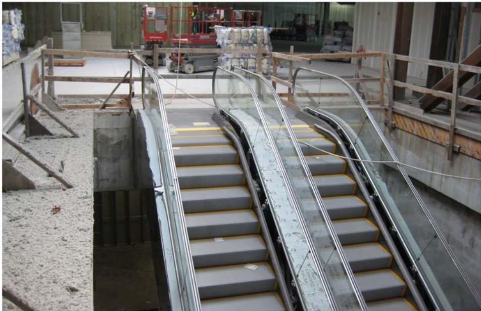
Miami Intermodal Center Construction: Progress Photo February 13, 2009 Rental Car Center (RCC): FM # 249937-5 Construction of RCC Lobby / Vertical Circulation
