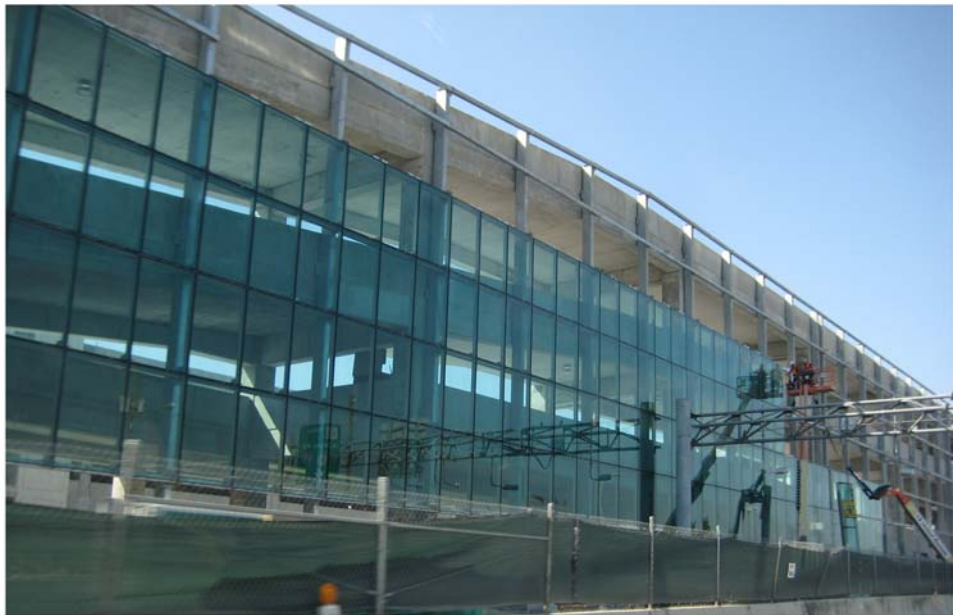
Miami Intermodal Center Construction: Progress Photo February 13, 2009 Rental Car Center (RCC) Lobby: FM # 249937-5 View of Curtainwall System on North Ramp along NW 25th Street
