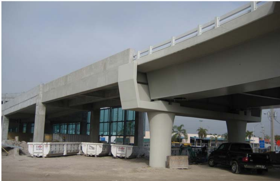
Miami Intermodal Center Construction: Progress Photo February 13, 2009 Rental Car Center (RCC): FM # 249937-5 / MTAR FM: # 249937-4 View of MIC Terminal Access Road Bridge 10-A
