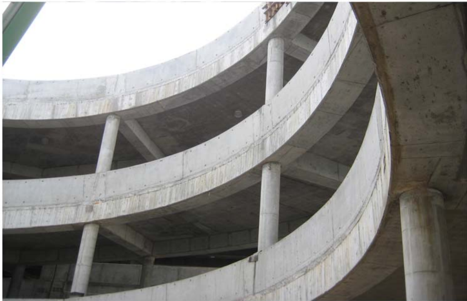
Miami Intermodal Center Construction: Progress Photo January 27, 2009 Rental Car Center (RCC): FM # 249937-5 View of Crash Walls on RCC North Helix Ramp
