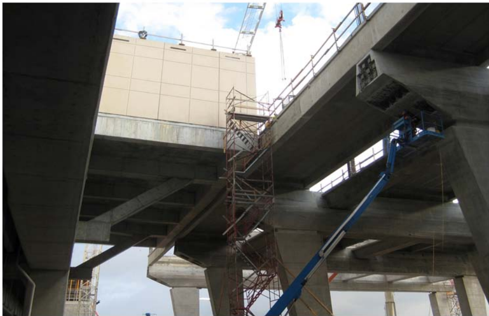
Miami Intermodal Center Construction: Progress Photo January 27, 2009 Rental Car Center (RCC): FM # 249937-5 / MIC-MIA Station: FM # 406800-6 Underside view of MIC-MIA Connector Station Straddle Bent, Platform, and U Beam
