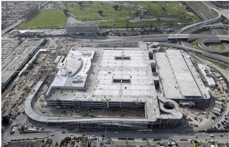
Miami Intermodal Center Construction: Progress Photo January 27, 2009 Rental Car Center (RCC): FM # 249937-5 Southwest View of RCC Construction Site
