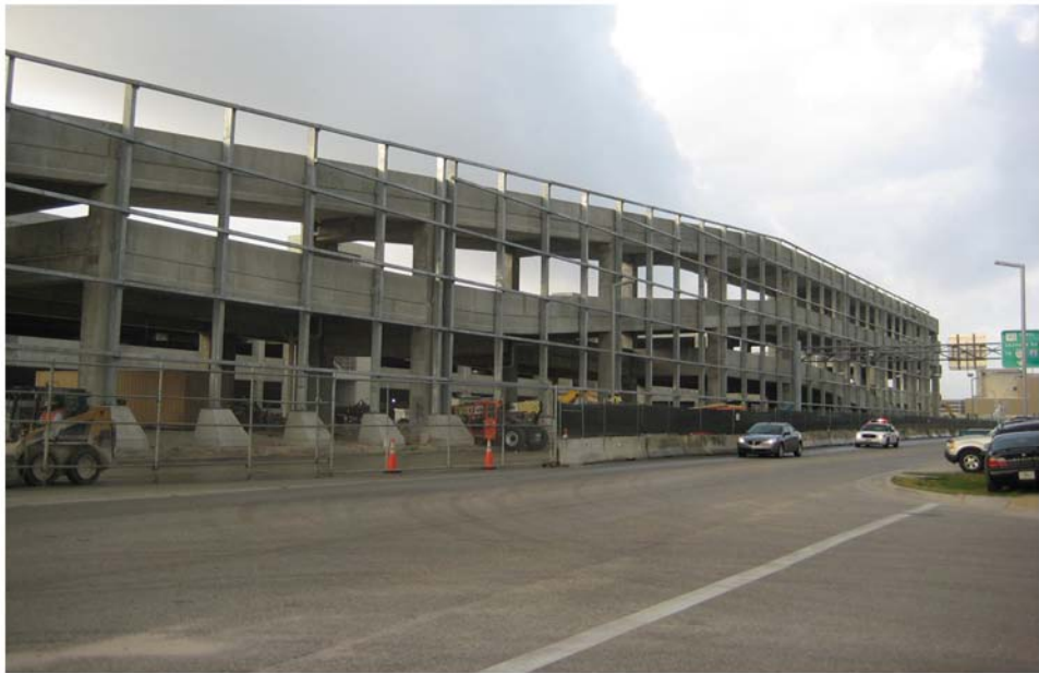
Miami Intermodal Center Construction: Progress Photo January 27, 2009 Rental Car Center (RCC) Lobby: FM # 249937-5 View of Curtainwall System on North Ramp along NW 25th Street
