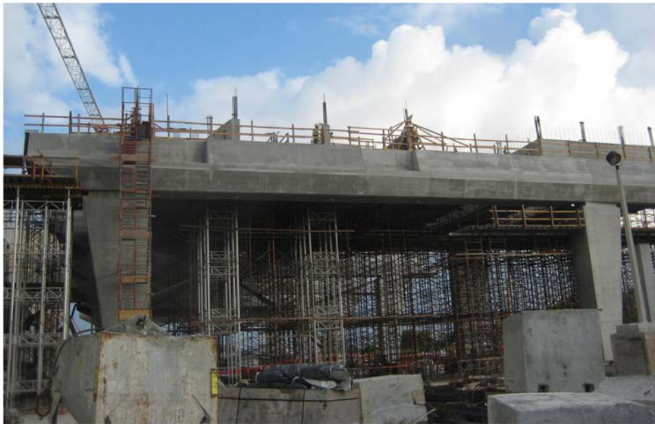
Miami Intermodal Center Construction: Progress Photo January 27, 2009 Rental Car Center (RCC): FM # 249937-5 / MIC-MIA Station: FM # 406800-6 Construction of MIC-MIA Connector Station Straddle Bent
