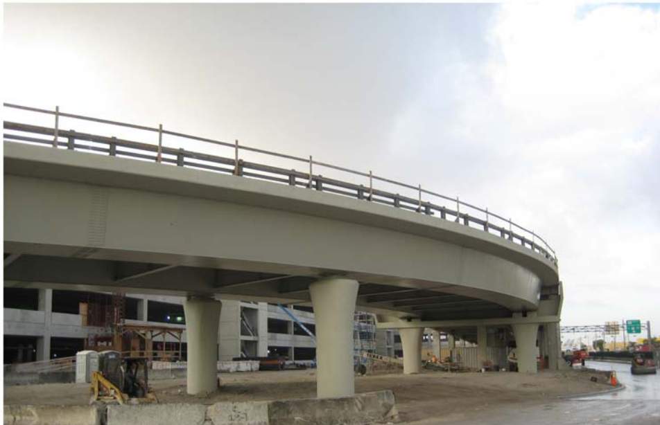
Miami Intermodal Center Construction: Progress Photo January 27, 2009 Rental Car Center (RCC): FM # 249937-5 / MTAR FM: # 249937-4 View of MIC Terminal Access Road Bridge 10-A
