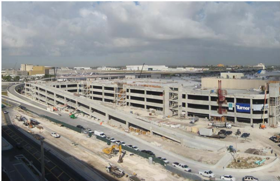
Miami Intermodal Center Construction: Progress Photo January 27, 2009 Rental Car Center (RCC): FM # 249937-5 / MTAR NW 21st Rd: FM # 249937-7 Construction of RCC South Ramp and Improvements to NW 21st Street
