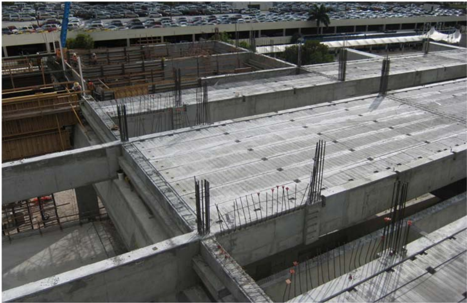
Miami Intermodal Center Construction: Progress Photo January 27, 2009 Rental Car Center (RCC): FM # 249937-5 / MIC-MIA Station: FM # 406800-6 View of MIC-MIA Connector Station Platform Construction
